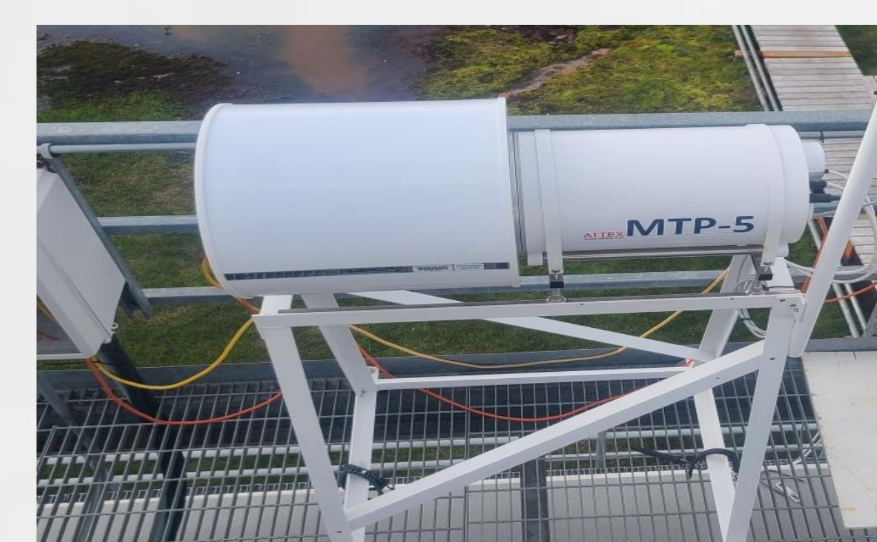
Figure 6: The MTP-5 Profiler installed at the NSA C1 site in Utqiagvik, Alaska.
